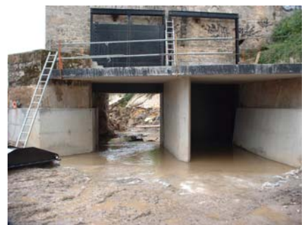
Water intake almost finished, valves in place and flapgate waiting to be placed
