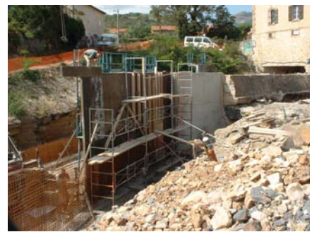
Sheeting of the side walls at the level of the VLH unit installation
