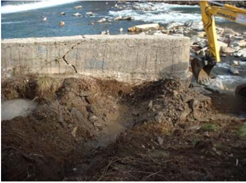
Cleaning and sounding downstream of the mill at the level of the VLH implantation
