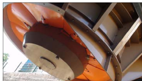
Bottom view of the Huningue lock #2 VLH In lifted position
