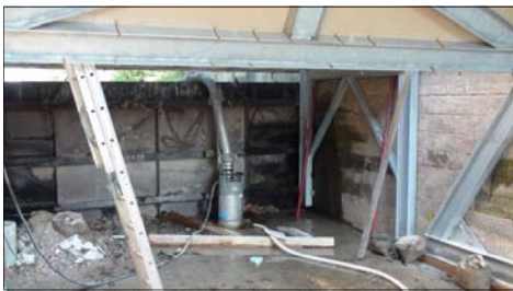
Metal supporting structure of the VLH and of the equipment room
