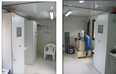
Electric equipment and equipment room
